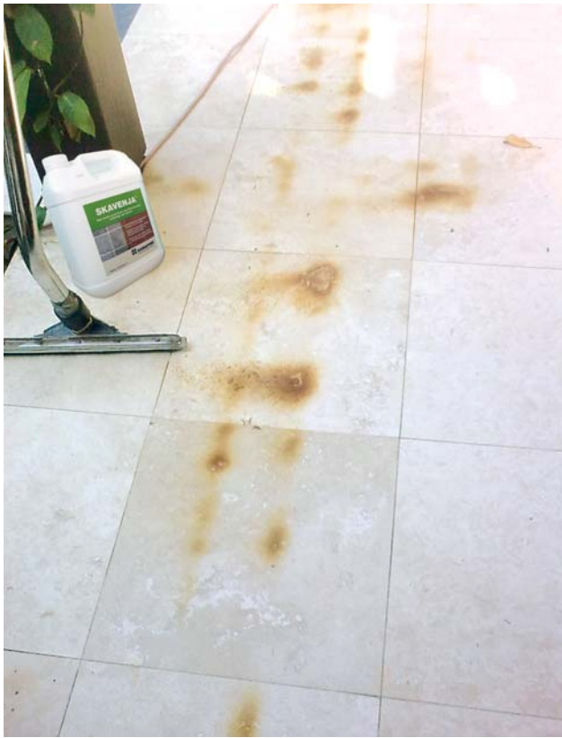
Rust stains before cleaning
