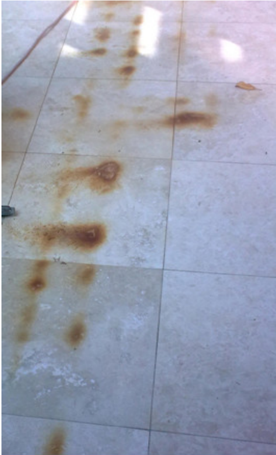
Rust stains before cleaning
