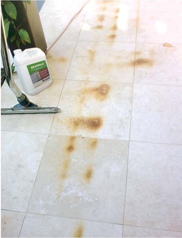
Rust stains before cleaning
